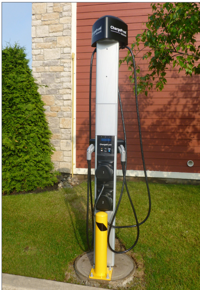
Figure 5. An EV charging station with cord management | Courtesy Energetics Incorporated
