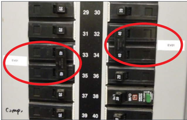
Figure 11. Level 2 Charging Station 240-volt (40 amp) circuits breakers and examples of empty breaker slots Courtesy Energetics Incorporated
