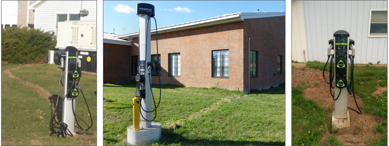
Figure 14. Charging stations can be installed by cutting and repairing (left and center photos) and tunneling under (right) concrete walkways Courtesy Energetics Incorporated
